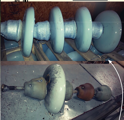
With rain comes lightning and many times lightning causes outages. Here are two pictures of transmission insulators before and after a lightning strike on May 29 th .
